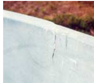
A crack caused by a failed glass joint, as shown above, usually starts small and grows rapidly.
