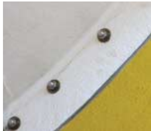
This image shows a stress crack, distinguished by a brown stripe near the bolts, on the backside of a flume.
