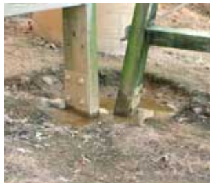
The footing above sits in a collection hole, exposing the vertical columns to excessive moisture.
