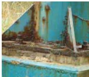
If not given proper attention, rusted and corroded steel columns and beams can lead to progressive deterioration of a slide's support structure. This image shows rust in the foundation as a result of overhead leaking.
