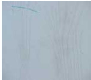
This is an example of early stress cracking in the gel coat.
