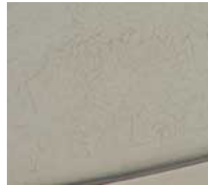
These surface cracks are caused by inappropriate coating over the fiberglass.
