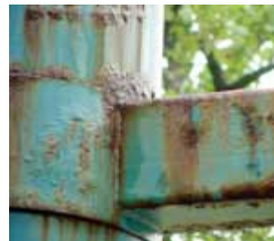
Visible stain lines run down this column.
