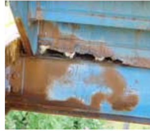
The underside of these steel steps exhibit the signs of a long period of neglect.
