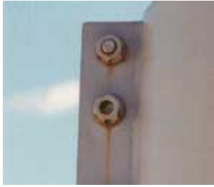
The bolts on the collar show signs of water trapped inside.
