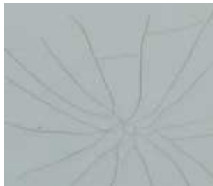
The classic star crack shown above is caused by an impact, such as a dropped tool or a sharp blow to the slide. If not attended to, the fiberglass will eventually chip or flake away.
