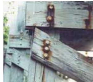
The deteriorating, rusted steel bolts and the cracks in the wood structure above deserve a structural evaluation.
