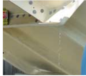
This is an example of a typical leak in a slide joint due to a gasket failure.
